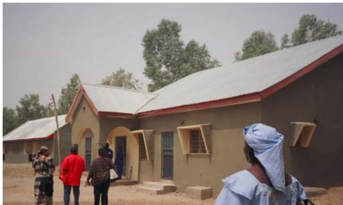
Rev. Donna Jones (EPA), Rev. Abinatuze, council director for UM Church of Nigeria (UMCN), and Rev. Hilda Campbell (EPA) stand near the orphanage in mid-construction. In the right foreground is Sister Fatima, also of UMCN.
